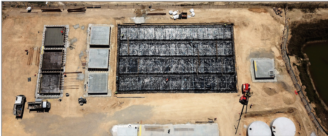
Works are taking place to build Tweed's new organic processing facility at the Tweed Resource Recovery and Landfill Centre at Stotts Creek.
