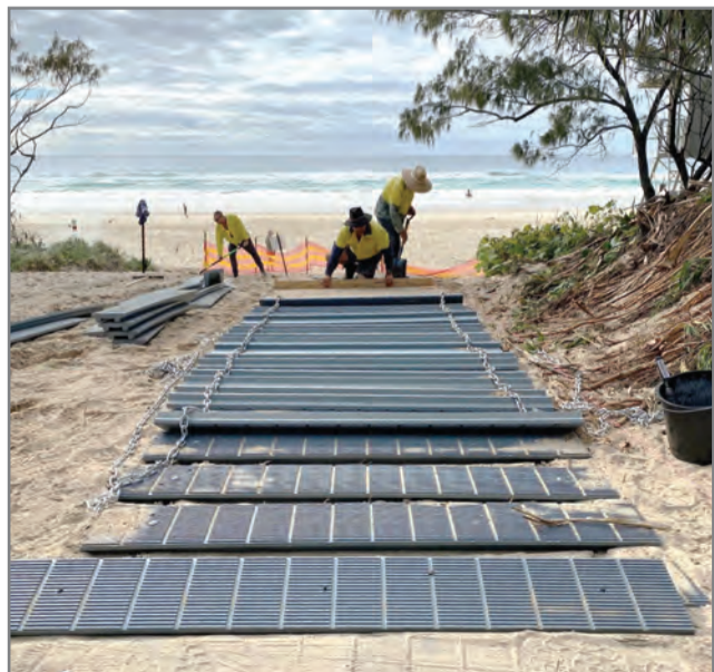
Recycled plastic planks are being trialled at a beach access at Salt.
