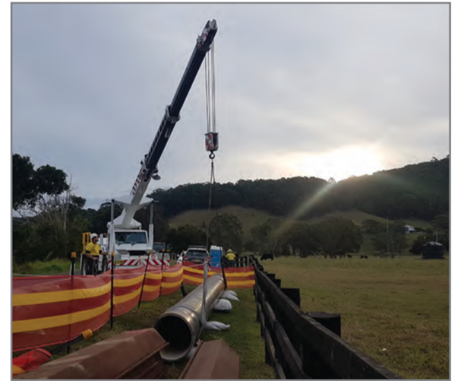
As the sun sets, the new pipe is ready to be lifted into place.
