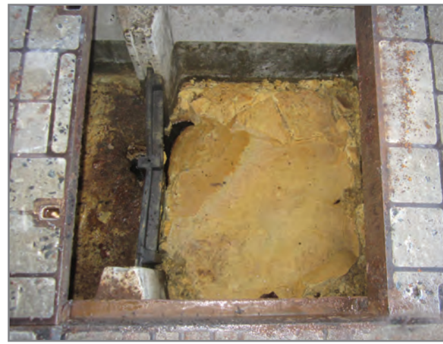
Council is offering to relax the frequency of grease trap servicing for businesses operating at reduced capacity.
