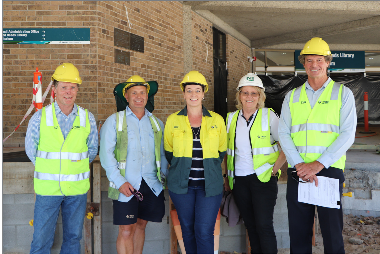
Some of the members of the Tweed Heads Civic and Cultural Centre redevelopment team inspecting the site are (from left) Warren Boyd, Paul Mitchell, Jacqui Turner, Joanne Watters and Todd Remmers.
