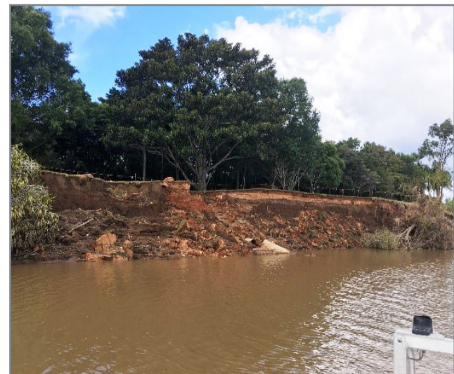
A section of the South Murwillumbah Levee damaged by the March 2017 flood.
