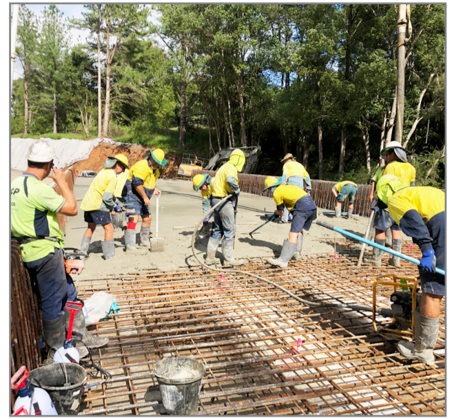
And on it goes – pouring the deck of the new Byrrill Creek Bridge.
