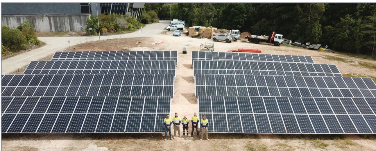
The team of installers from Nevmat Australia Pty Ltd near completion of Council's first ground-mounted solar array at Bray Park.
