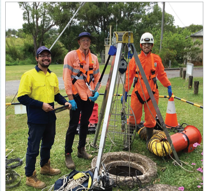
Environmental Services' Fabio Ortiz stands by as Lloyd Johnstone is harnessed up to enter the manhole and Manfred Faust stands ready if needed.
