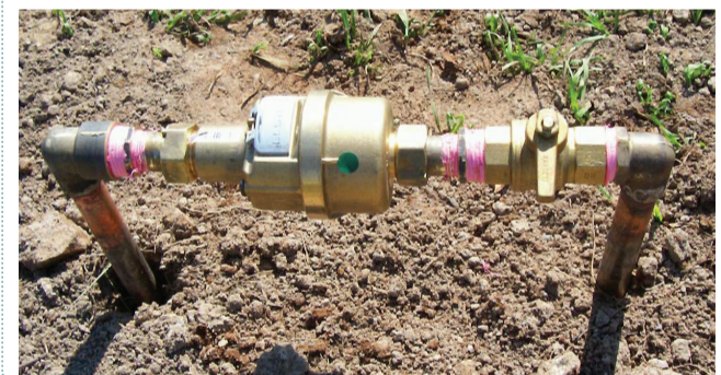
A newly installed above ground residential water meter.
