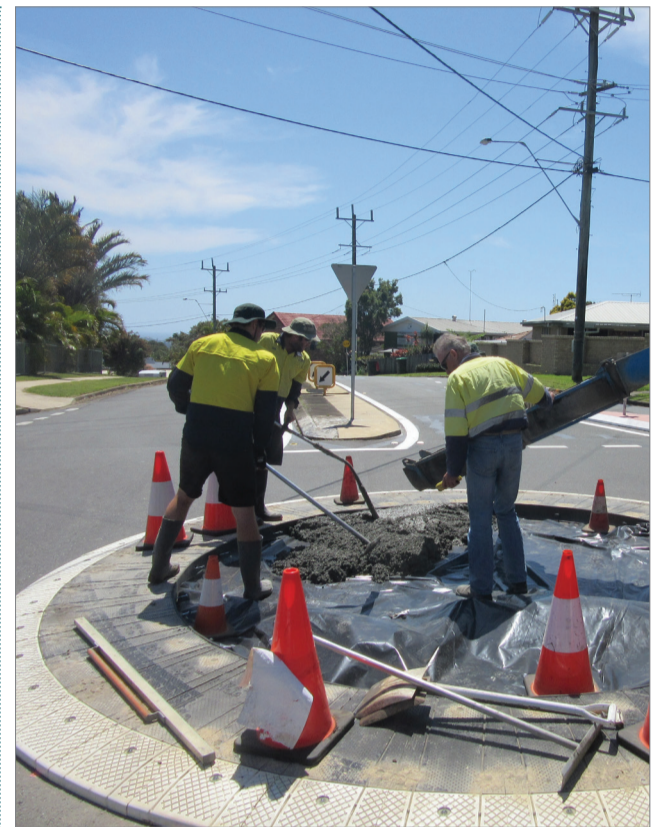
The Tweed's first rubber roundabout takes shape in Bilambil Heights last week. The roundabout was installed within one day at the corner of Bilambil Road/Scenic Drive and McAllisters Road/Simpson Drive at a cost of $25,000.
