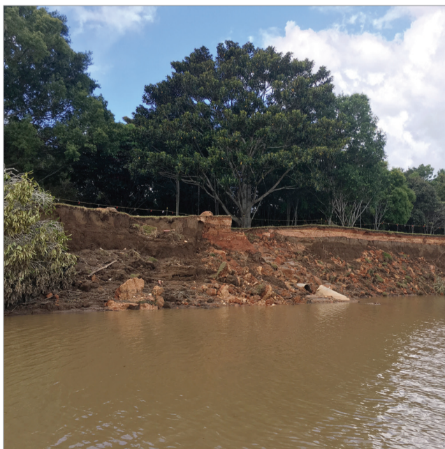
The South Murwillumbah levee at the river's edge was severely damaged in the March 2017 flood.
