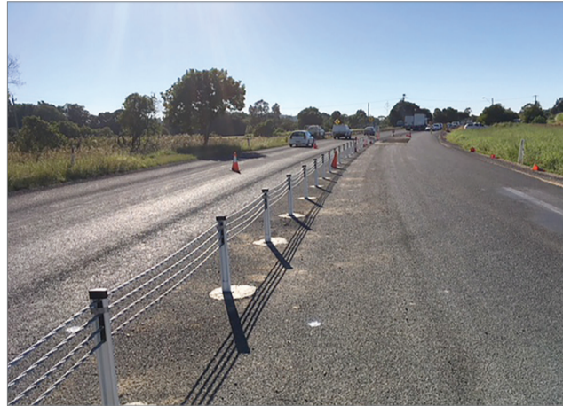
The wire rope median on Tweed Valley Way between the two Riverside Drive entrances to the village of Tumbulgum.
