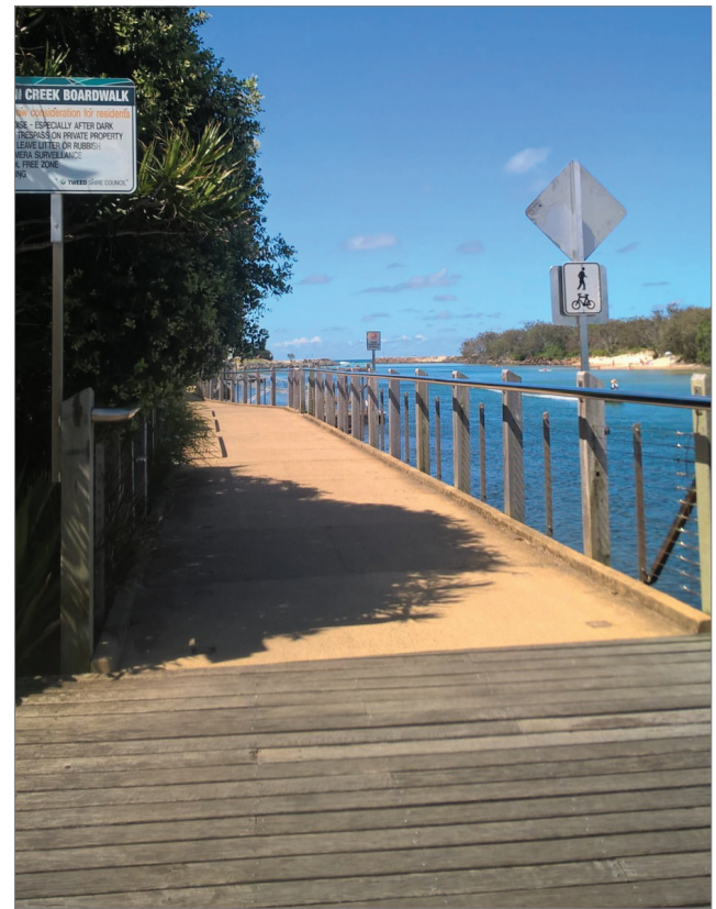
The old and the new. The final section of timber boardwalk will be replaced with a concrete shared-user path.
