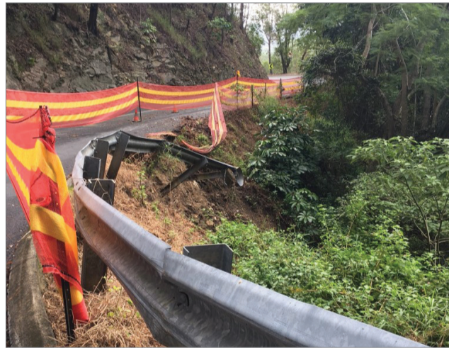
The site of the major landslide on Clothiers Creek Road.
