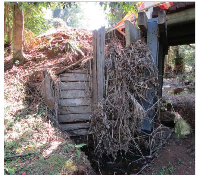
The photograph does not show the real extent of the damage of this bridge on Geles Road at Upper Burringbar. The abutment needs to be replaced, the wing walls stabilised and repaired, the concrete apron reinstated and then the road approaches repaired.
