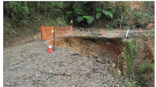
Some of the flood damage on Cudgera Creek Road.
