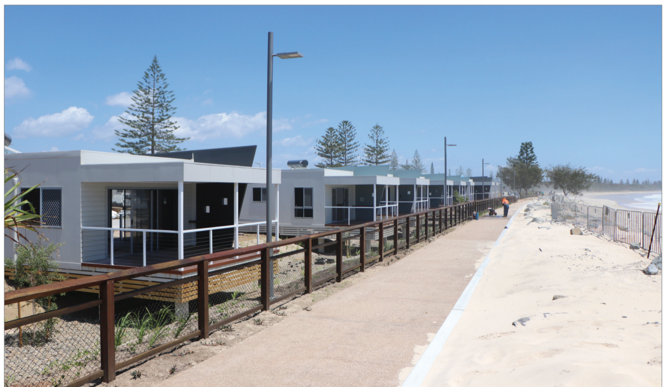
The new holiday park at Kingscliff takes shape with cabins facing the beach. Central Park is completed and is awaiting commissioning of the electricity supply for various components before it can open to the public. By that time, Marine Parade's tourist strip will have a shiny new road surface.
