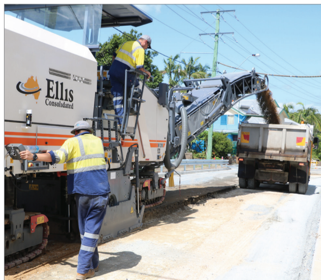
Contractors mill off the old road pavement in preparation for a new temporary seal, ahead of the final pavement which will go on before the end of February, weather permitting.
