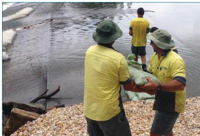
Workers last week prepare to sandbag the wall of the weir to protect it from overtopping in this week's high tides.
