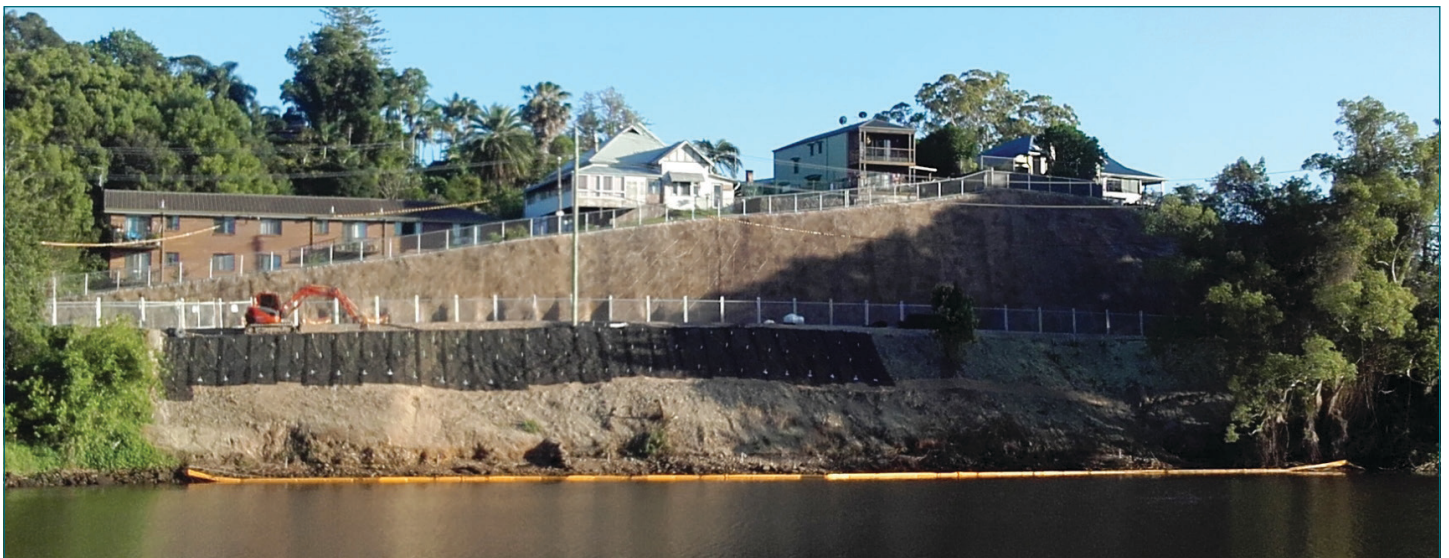
The view from across the river shows the depth of the embankment and the scope of the riverside stabilisation works. Jute matting will be placed below the mesh and wire shown above.
