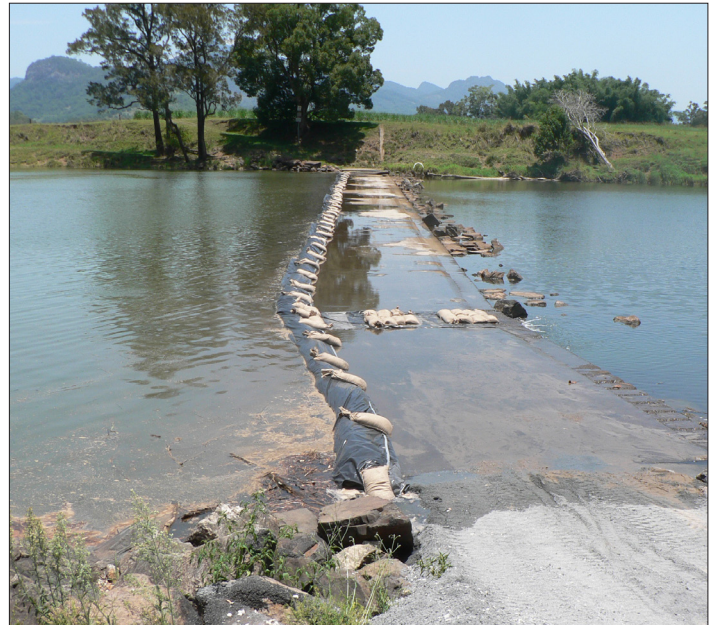
The Bray Park Weir wall is usually sandbagged when very high tides are expected. Unfortunately, the predicted peak was well exceeded last Monday, and salt water entered the weir pool.
