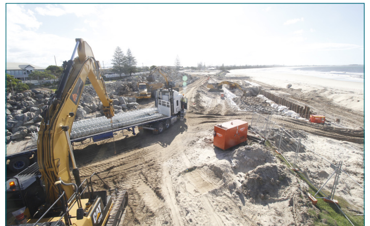
Laying the initial rock bed at the northern end of the site.
