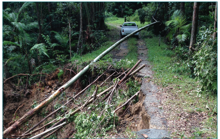
A large section of Lone Pine Road at Doon Doon washed away.
