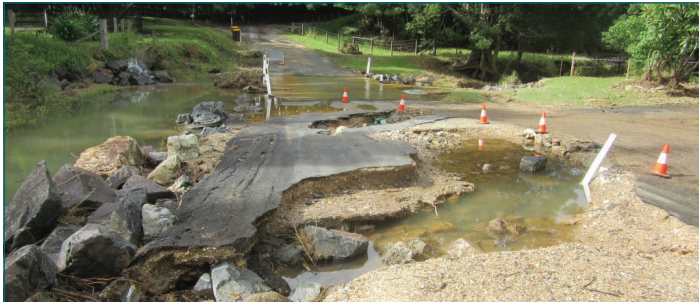
Damage to Dungay Creek Road was clearly visible once the flood water receded, clear evidence to never enter floodwater.
