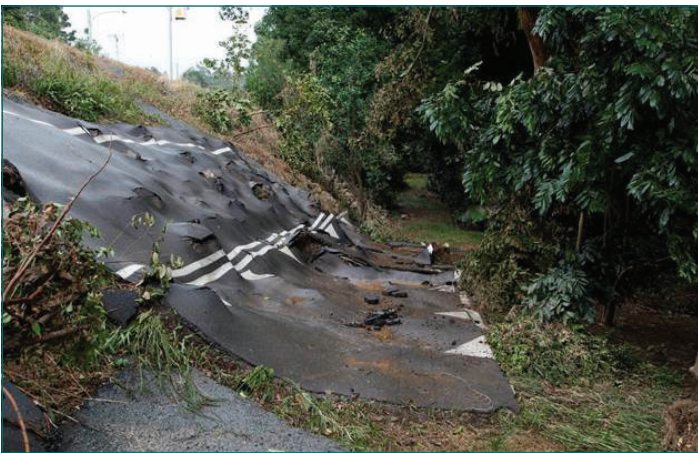
Part of the road surface at Uki just slipped away.
