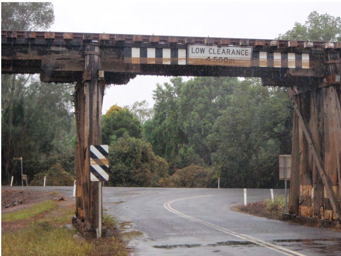
Wilson's River, Winterton Parade North Lismore 12.39pm 4 April 2017 debris line on bridge
