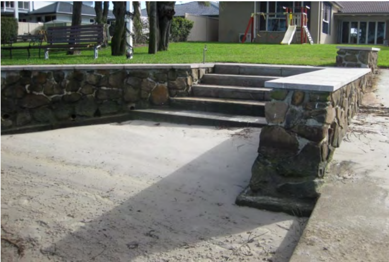
Figure 3: Existing near-vertical rock and concrete retaining wall, stairs and boat ramp adjacent to 20 Wyuna Road.
