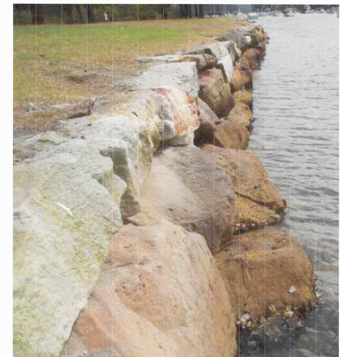
BOULDER RETAINING WALL (FIG. 22) SOURCE: ENVIRONMENTALLY FRIENDLY SEAWALLS OFFICE OF ENVIRONMENT AND HERITAGE (2012)
