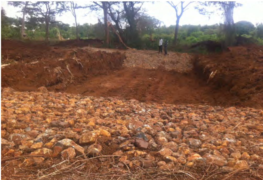
Figure 17: The newly constructed sediment trap located on the eastern side of dam
