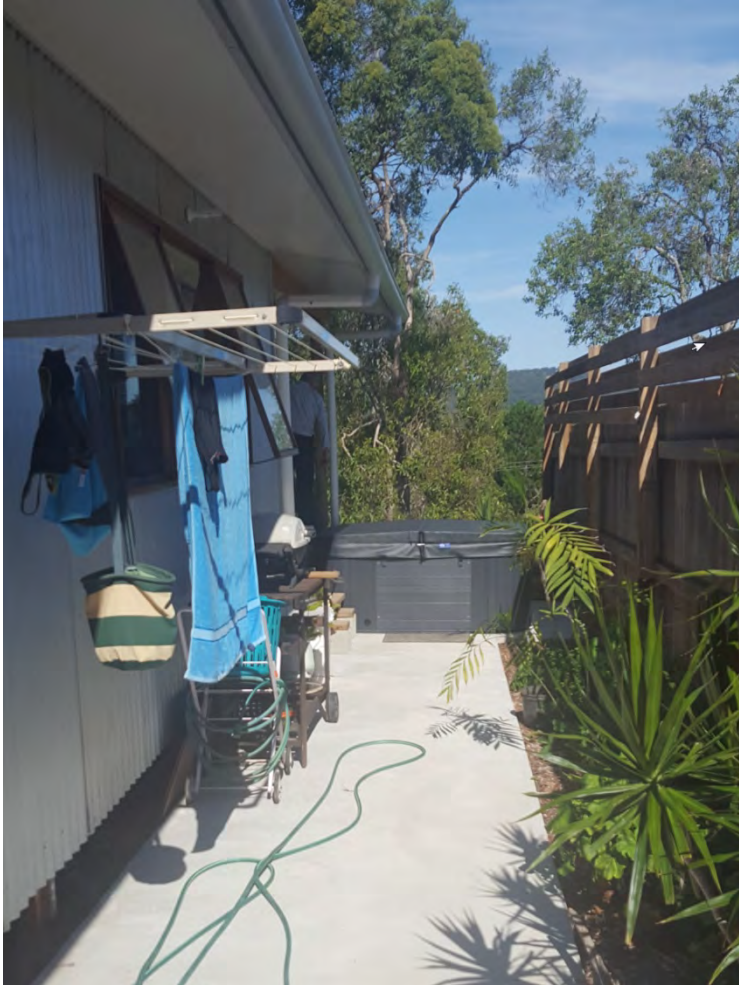
External Spa located on boundary which does not meet the exempt provisions
