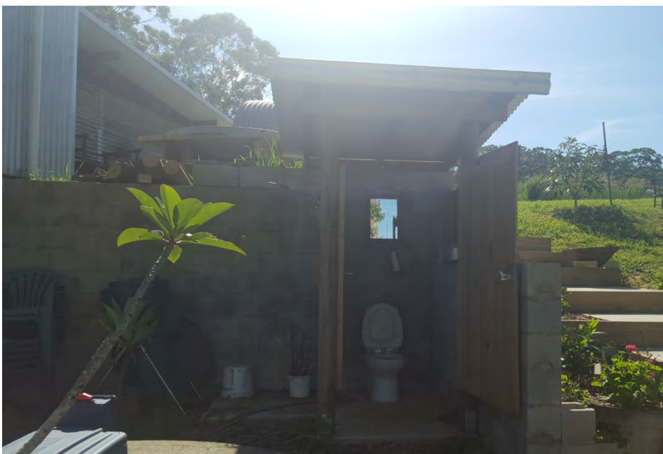
External Toilet and retaining wall erected without approval
