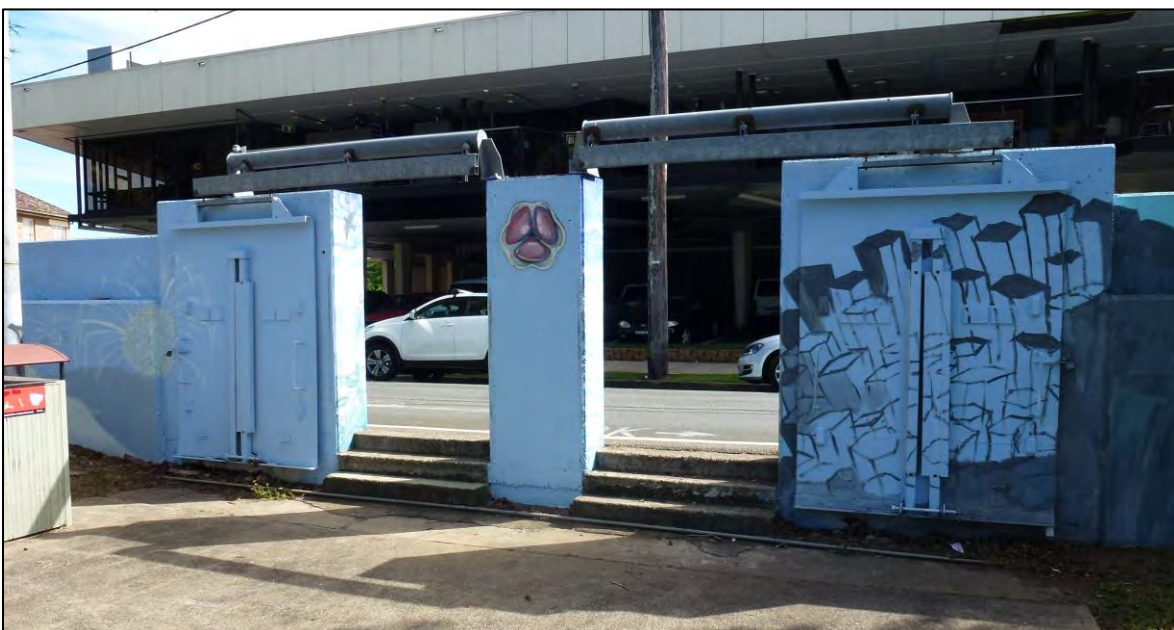
Plate 2 View looking west towards Murwillumbah Services Club showing concrete panel section of the Commercial Road levee with gated openings
