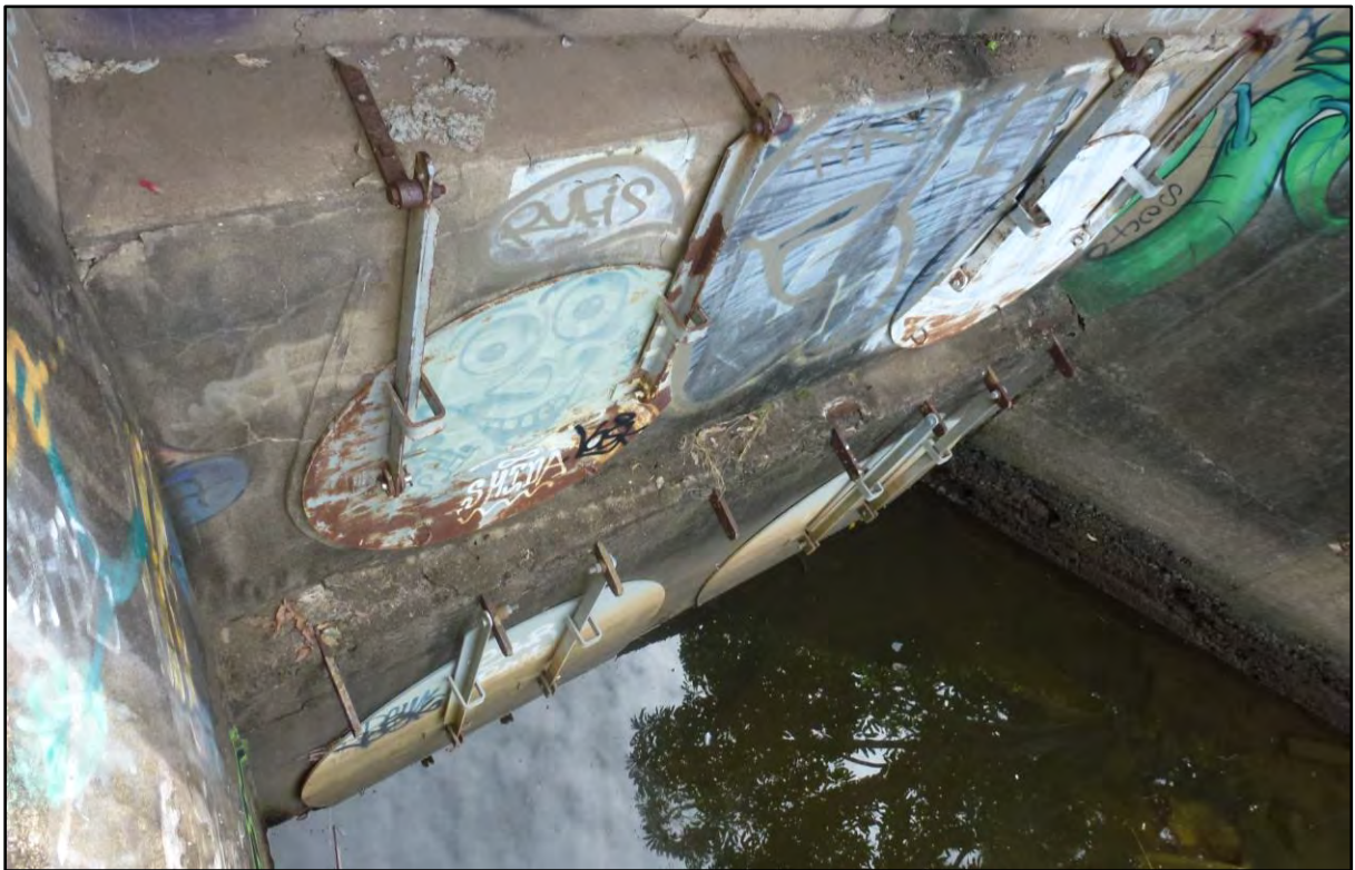
Plate 4 View showing flood gates on Tweed River side of Commercial Road culverts. The gates prevent water from the Tweed River “backing up” the culverts and inundating areas behind the levee
