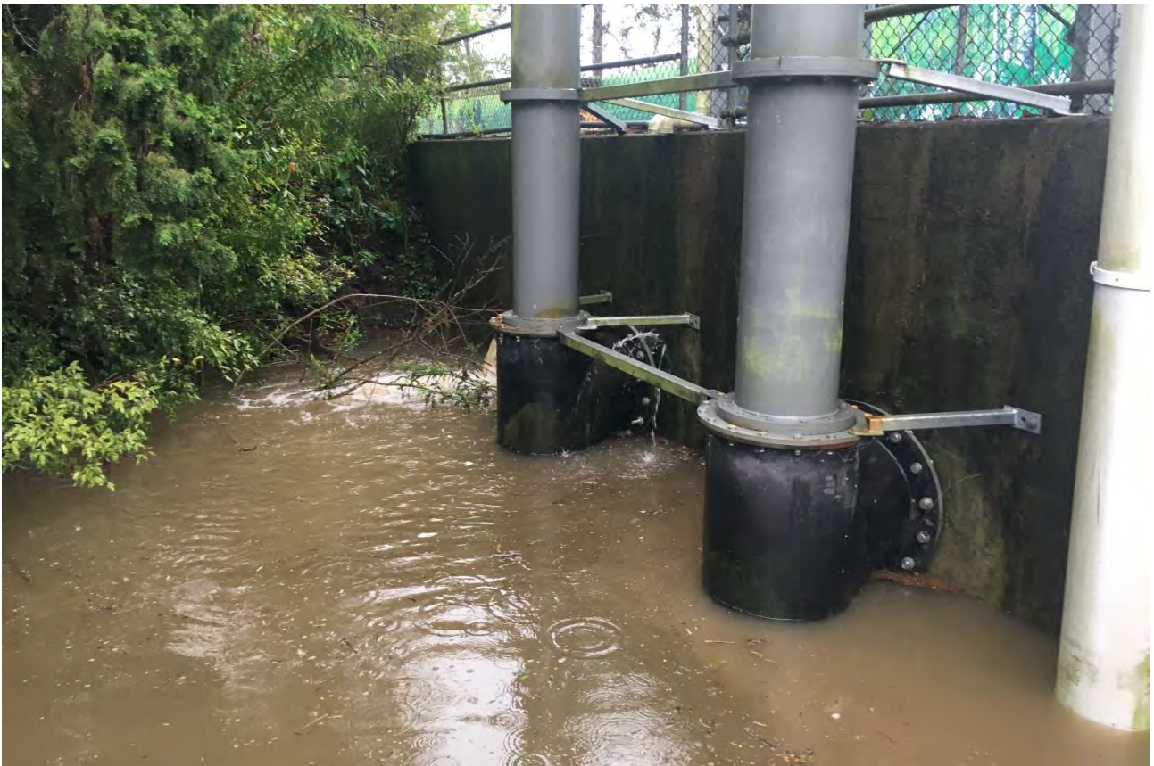
Lavender Creek Pump Station (3:00pm on 31 March 2017)
