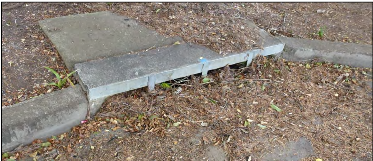
Plate 7 View showing partial blockage of a stormwater pit near Knox Park
