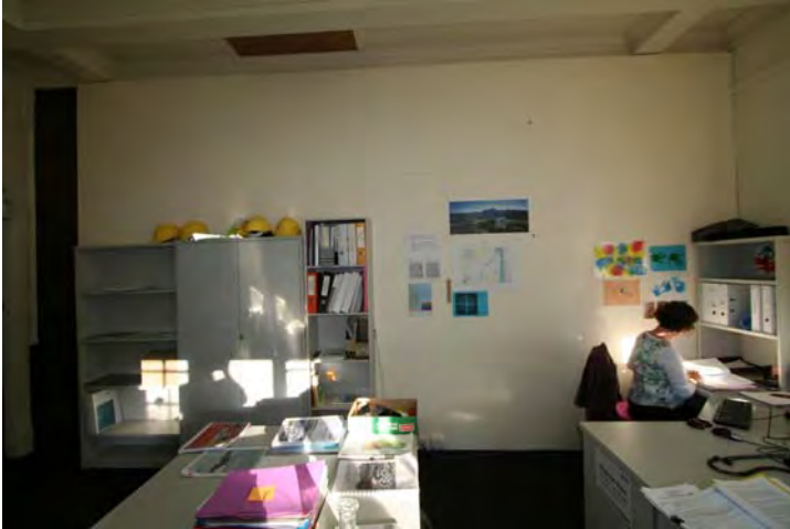
Photograph 88 A replaced partition wall after Gallery moved out does not quite meet the ceiling.
