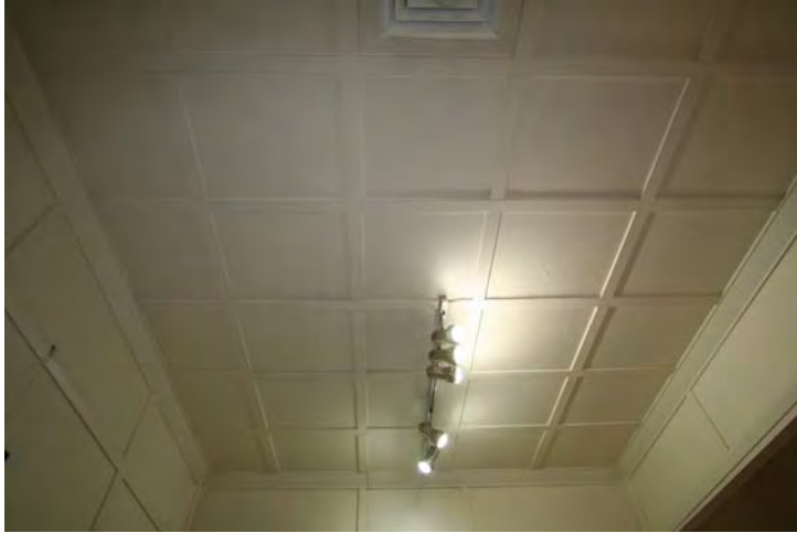
Photograph 109 The distinctive ceiling, cornice and bulkhead and the ineffective former gallery lighting
