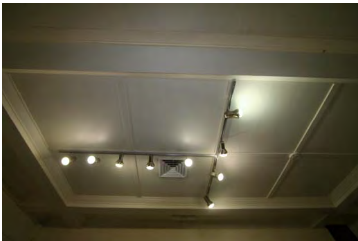
Photograph 77 The existing Exceptional ceiling with distinctive bulkhead and the former gallery track lighting which detracts from the heritage significance and is not efficient for the current use
