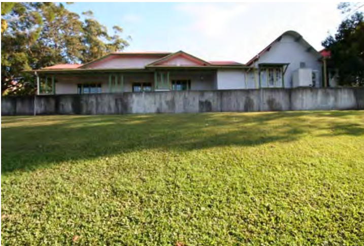
Photograph 50 The extension: Original fabric and Extension fabric and details – Moderate & Intrusive significance
