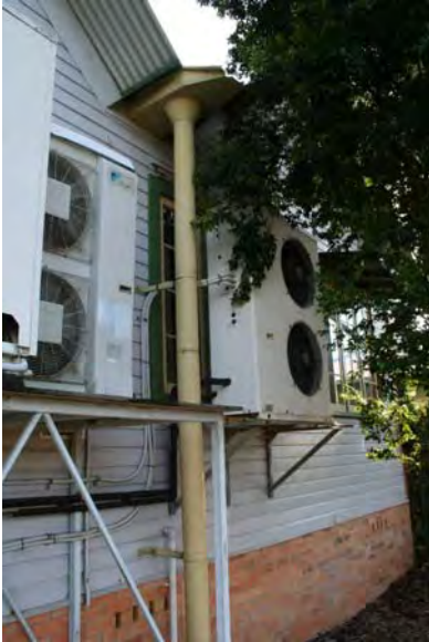
Photograph 28 Services on riverfront elevation - Intrusive
