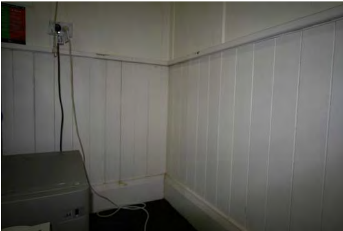
Photograph 92 Unusual half timbered dado area within the secondary and service areas of the former residence
