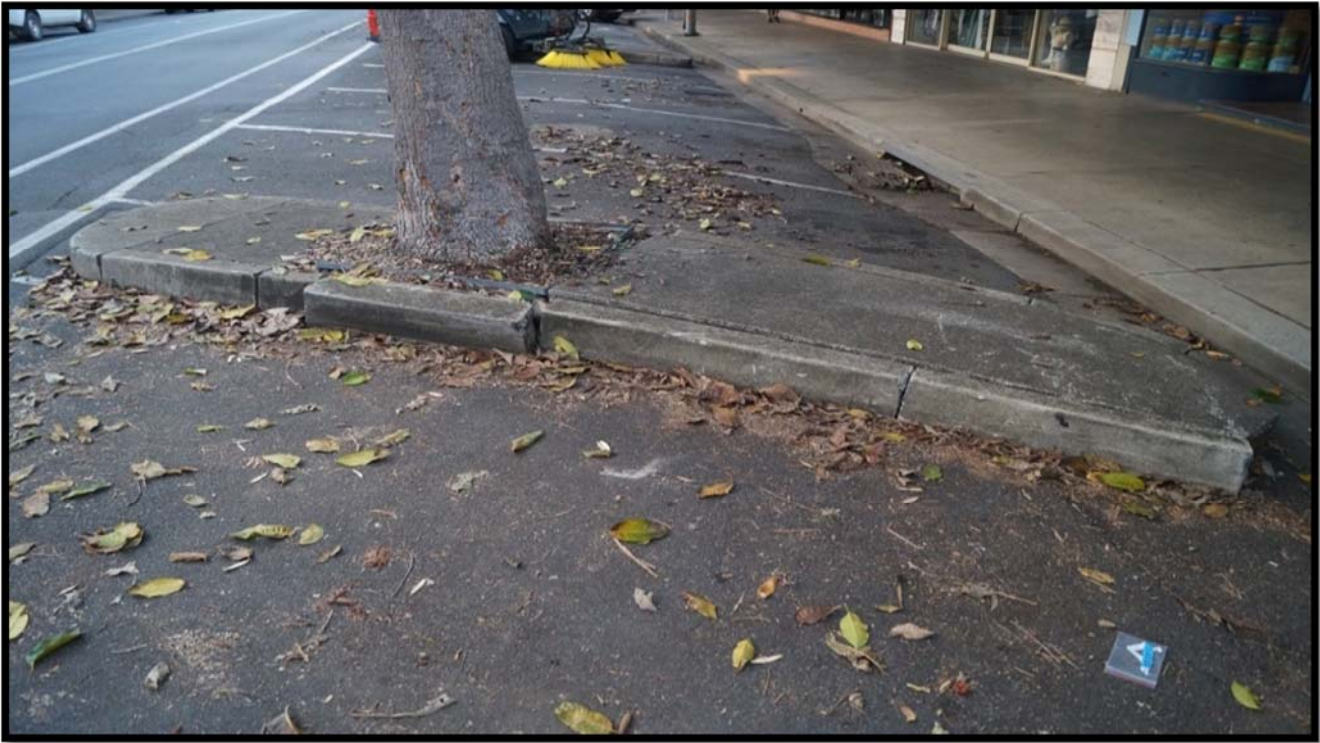
Photos- Infrastructure damage throughout the CBD Murwillumbah
