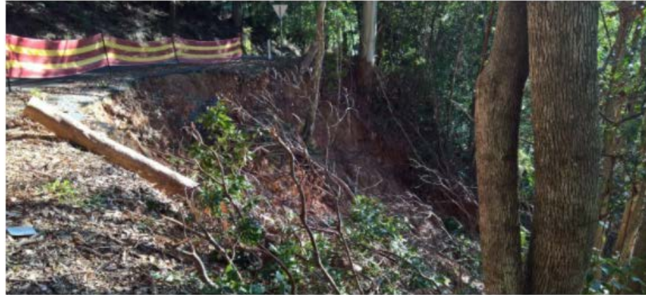
Photo 1: View looking north across the landslide area
