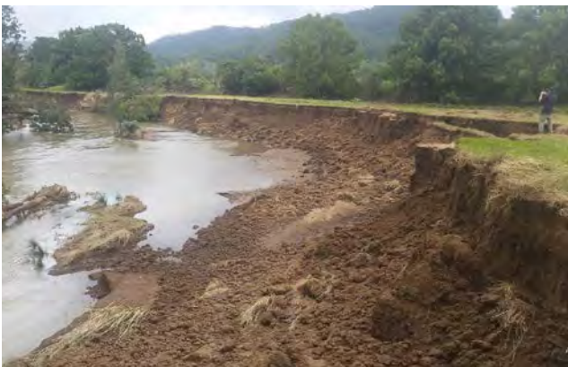
River bank erosion after March flood event, Oxley River.
