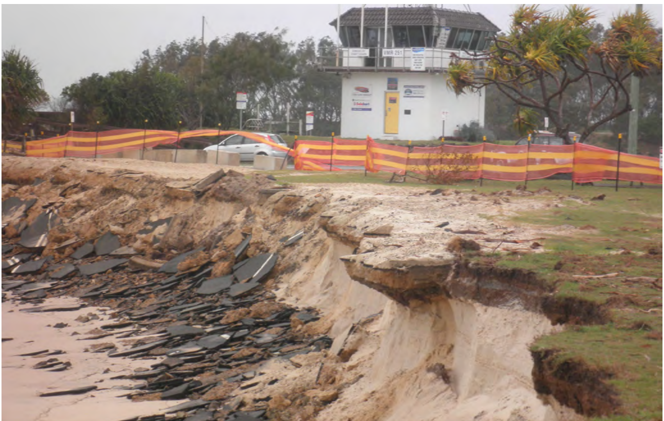
A storm in 2009 caused a significant erosion event along Kingscliff Beach.
