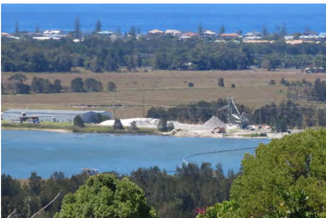
A sand extraction operation within the foreground with the future potential development site of North Kingscliff in the background.
