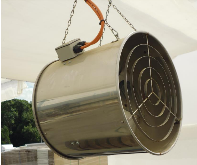
Photograph 1: Existing fans used in the facility
