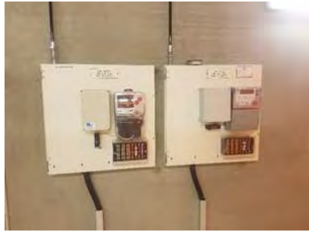
2 x utility meters at the site
