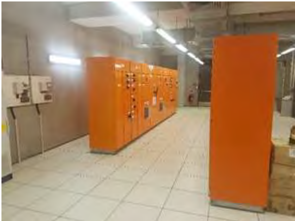
Main switch room with potential inverter location
