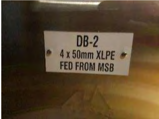
Feed to distribution board at eastern end top floor
