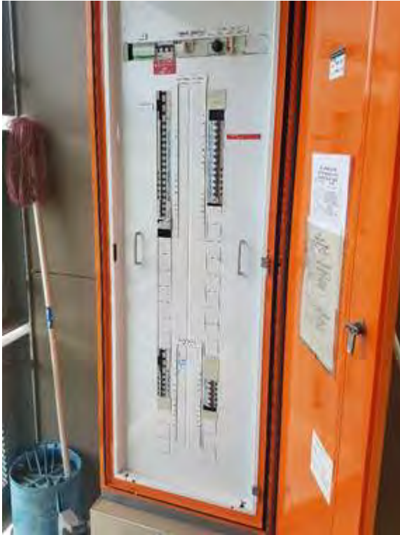
Distribution board in main building – space adjacent for inverters
