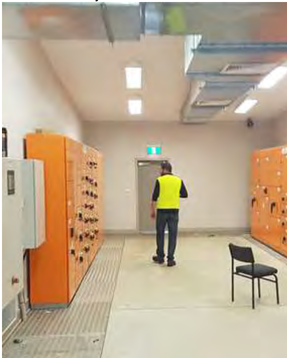
Main switch room with space for inverters as required
