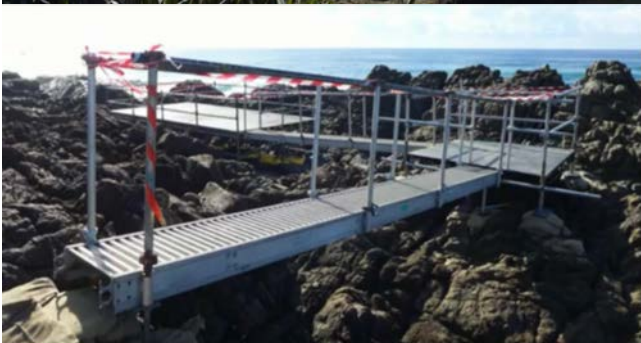
Photos of the temporary jetty constructed over the rocky foreshore (now removed)
