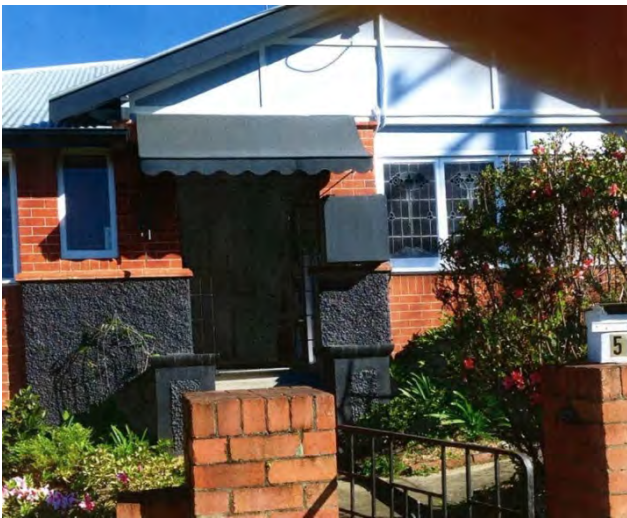
Front of house (Condong St) before with inappropriate black rendering to stucco
