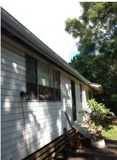
Rusty guttering to side of house after
