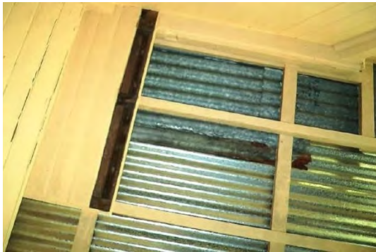
Damaged and leaking roof before
