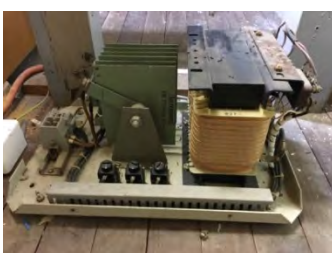
Aging transformer before
