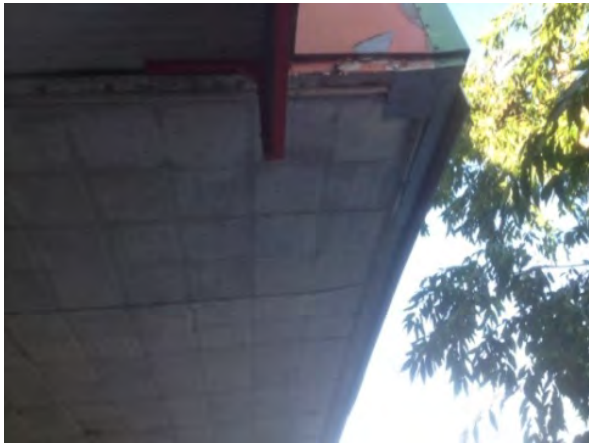
Rusted awning before
