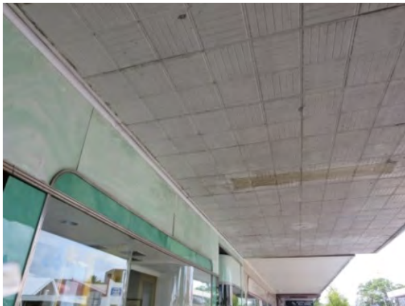
Rusted awning before
