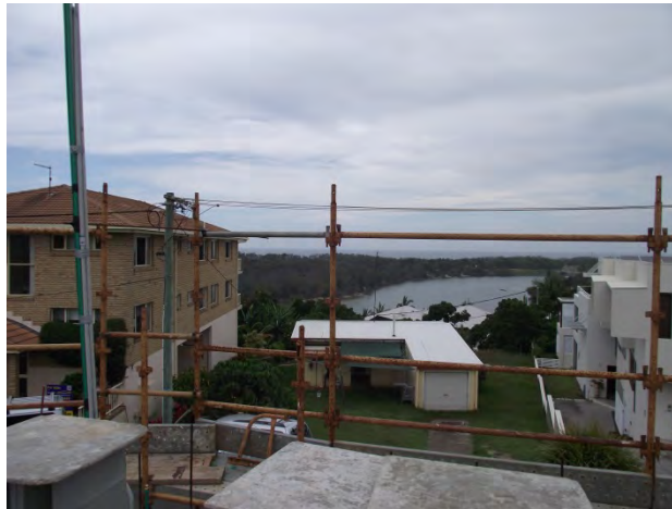
Photograph taken from upper level of dual occupancy currently under construction at 1 Hungerford Lane.
