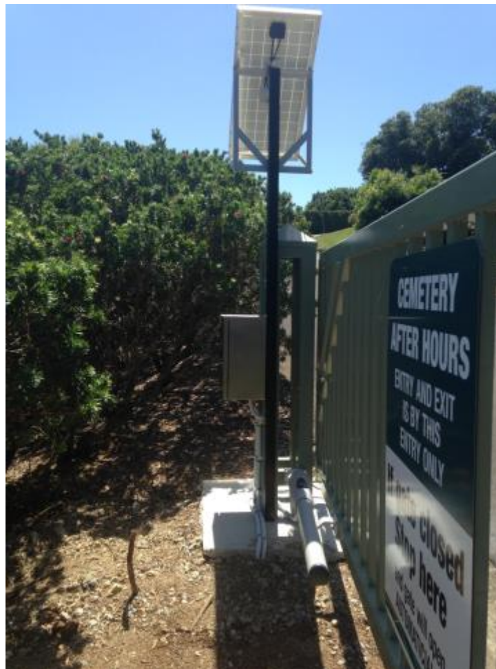
Figure 5 - solar powered self-opening gates installed at the Eviron cemetery
