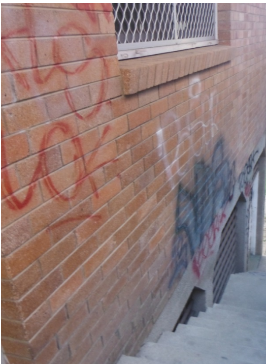
The walls of the CWA building next to the stairs going down to the rear car park
