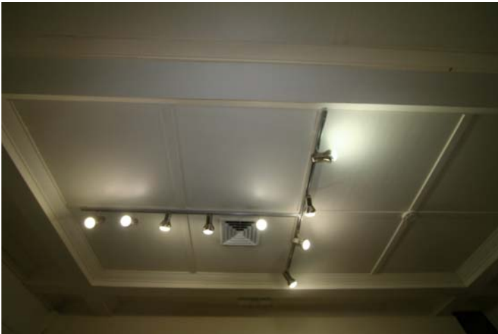
Photograph 77 The existing Exceptional ceiling with distinctive bulkhead and the former gallery track lighting which detracts from the heritage significance and is not efficient for the current use
