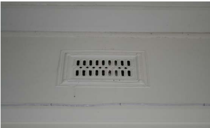
Photograph 128 Rare pressed metal wall vent and exposed conduit/wiring
