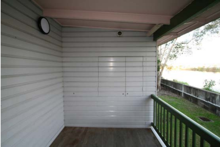
Photograph 73 Kitchen servery to the Southern verandah from early room modified for kitchen
