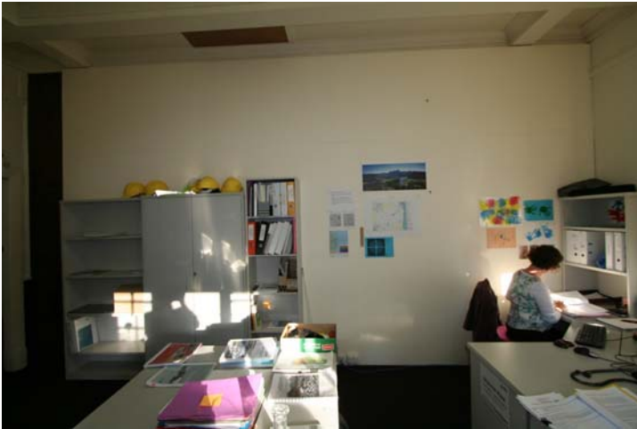
Photograph 88 A replaced partition wall after Gallery moved out does not quite meet the ceiling.
