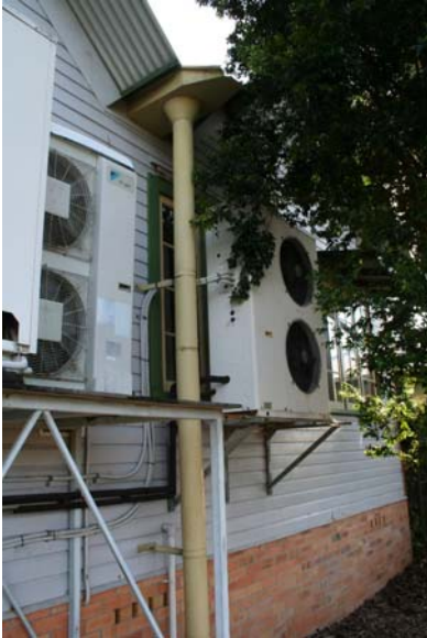
Photograph 28 Services on riverfront elevation - Intrusive
