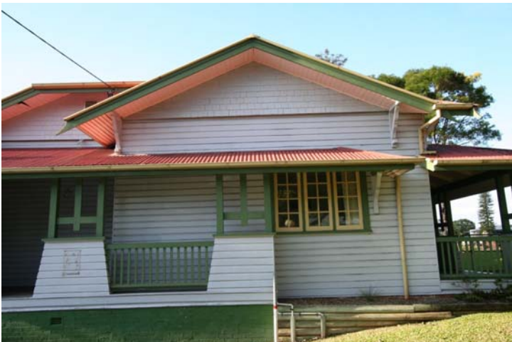
Photograph 63 Exceptional significant and exposed conduit and cables
