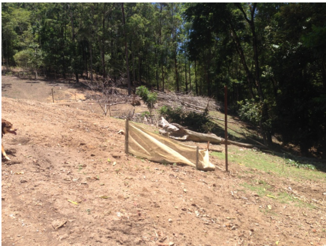
Photograph 4 - Demonstrates sediment and erosion controls have been installed along the exposed slope adjacent to the tributary that ultimately flows to Jacksons Creek.
