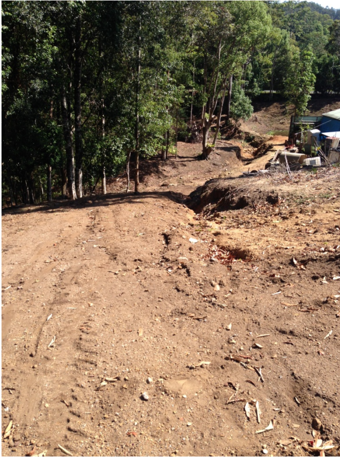
Photograph 2 - Drainage line adjacent to water course that improved sediment and erosion control practices were identified to be established.
