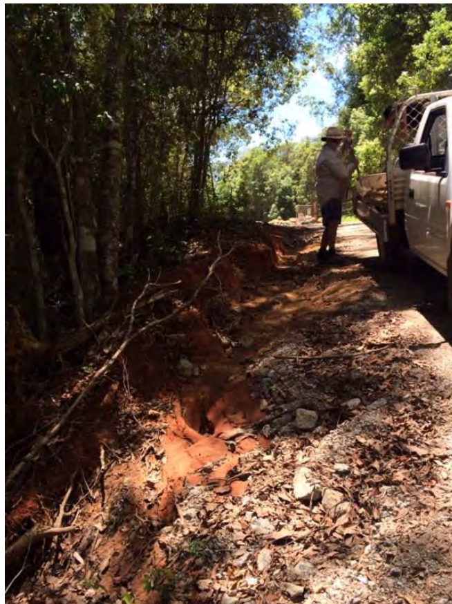
Photograph 8 - Provided by site owner to NSW Crown Lands 5 January 2015. Indicates top soil being installed prior to laying of turf near the entry gate.
