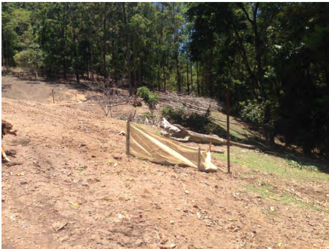
Photo 4 - Demonstrates sediment and erosion controls have been installed along the exposed slope adjacent to the tributary that ultimately flows to Jacksons Creek.
