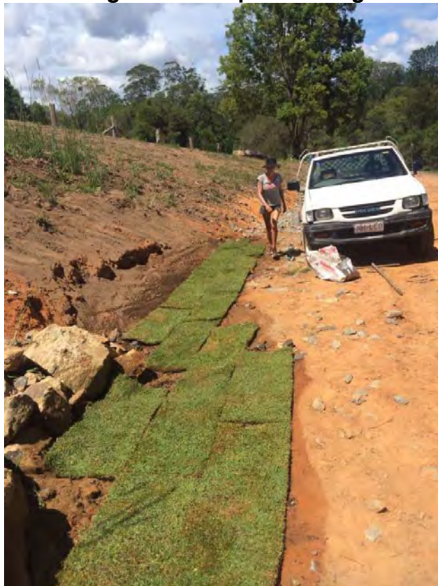
Photograph 10 - Provided by site owner to NSW Crown Lands 5 January 2015. Indicates turf has been laid along the house pad drainage channel.
