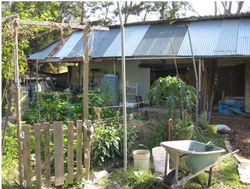
This is an unwired, unplumbed, unlined rural shed.
