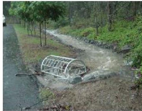
Diversion banks can be effective in diverting water from infrastructure.
