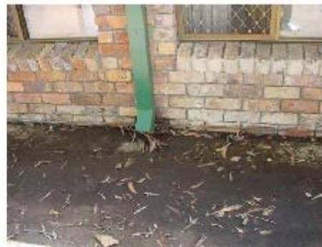
Roof gutters not connected to approved stormwater outlets can cause damage to your property and neighbouring properties
