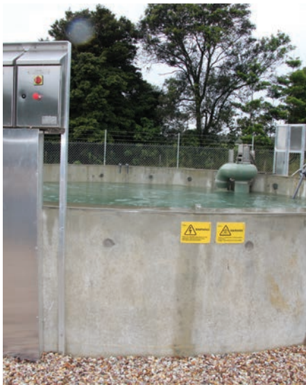
Burringbar-Mooball sewerage treatment plant
