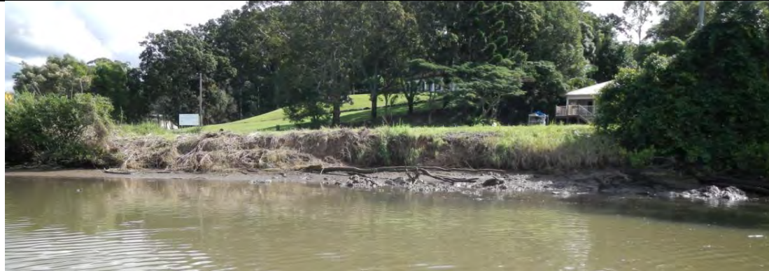
Photo 267– Bank erosion on downstream end of this site.
