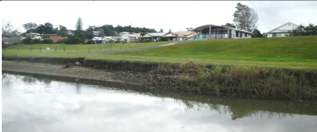
Photo 113 – showing minor erosion along bank toe
