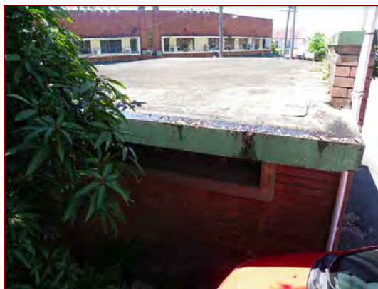
Figure 3.9: North elevation showing cracking of roof slab.
