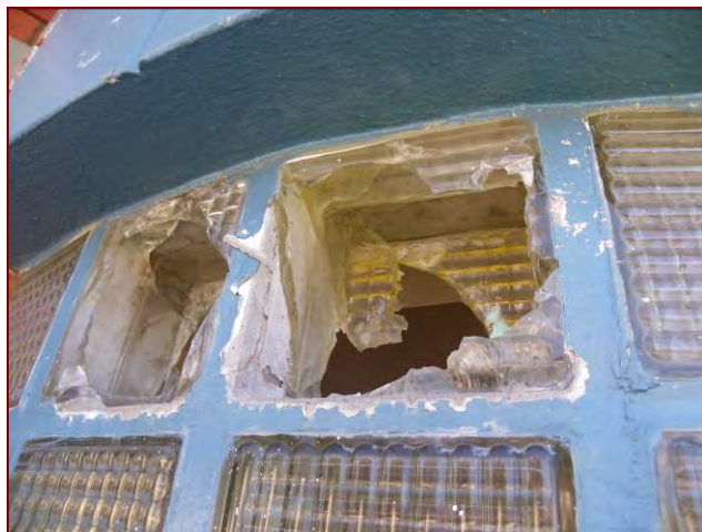
Figure 3.16: Broken glass bricks on the south elevation.
