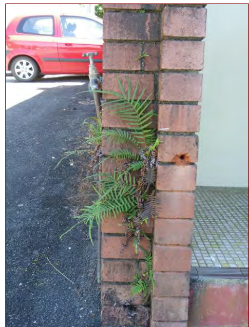
Figure 3.17: Damaged bricks and vegetation on the south elevation.
