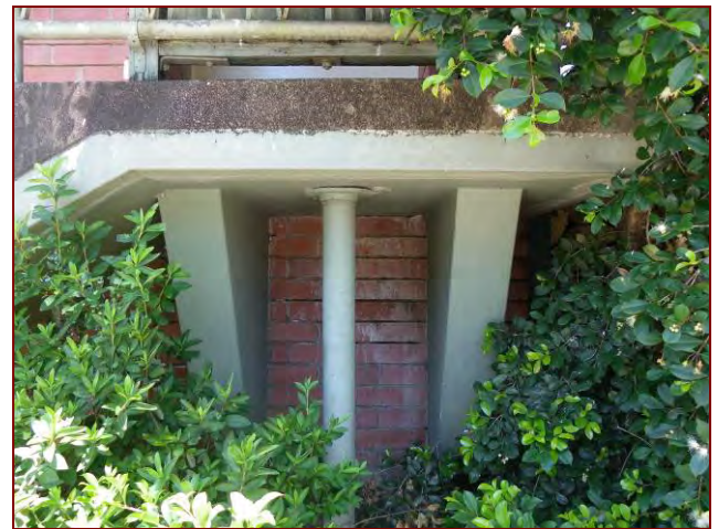
Figure 3.13: The stair supports, with later steel support. Water damage can be seen on the bricks behind.
