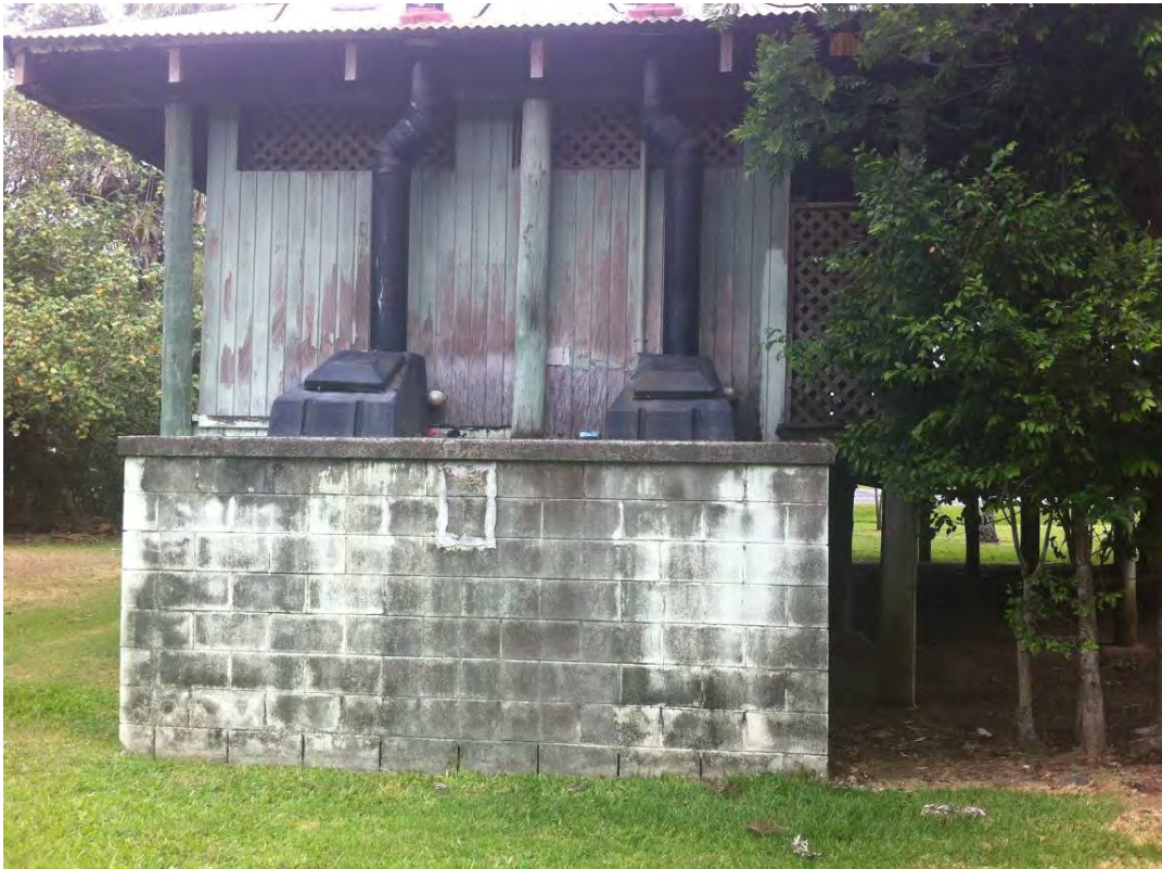
Photo 7 Existing waterless composting toilet, showing aboveground masonry chambers and plastic covers and vents.
