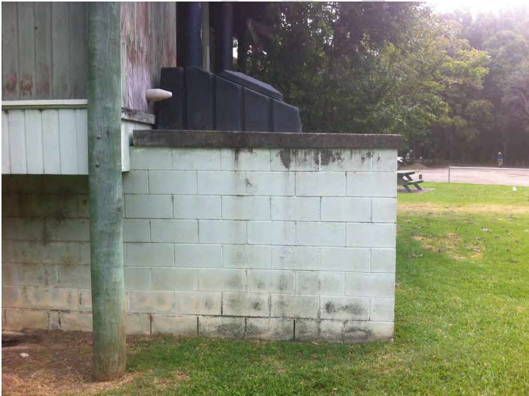
Photo 8 View from side of composting chamber showing clearance floor level clearance of 1.8m above ground level.
