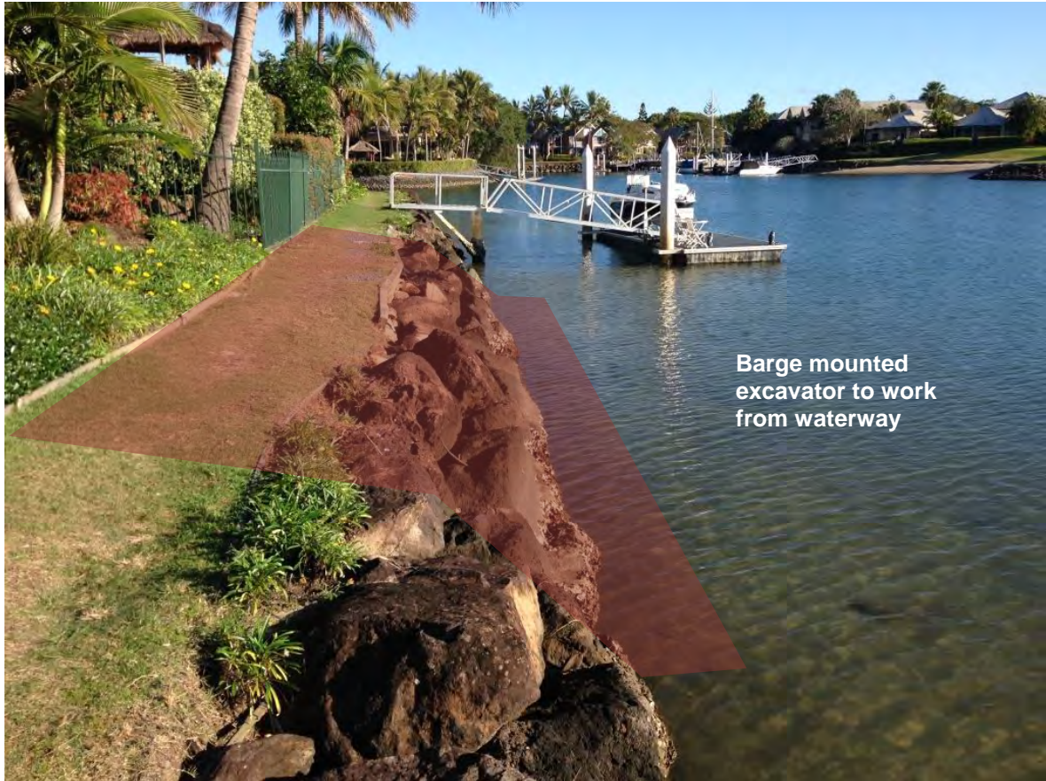
Plate 2: View looking south showing revetment repair site (works to be performed from the adjacent Terranora Inlet)
