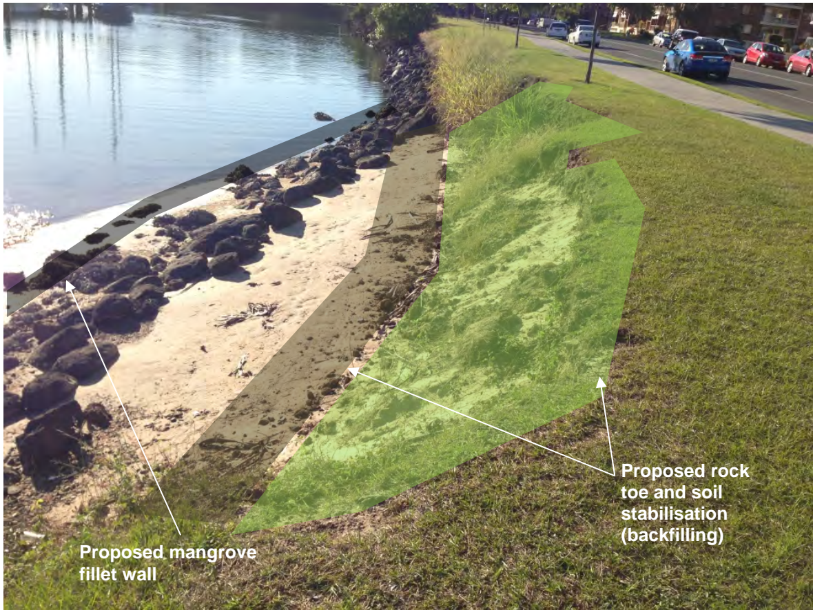
Plate 1: View looking north showing the road reserve bank slip stabilisation site adjacent Terranora Inlet
