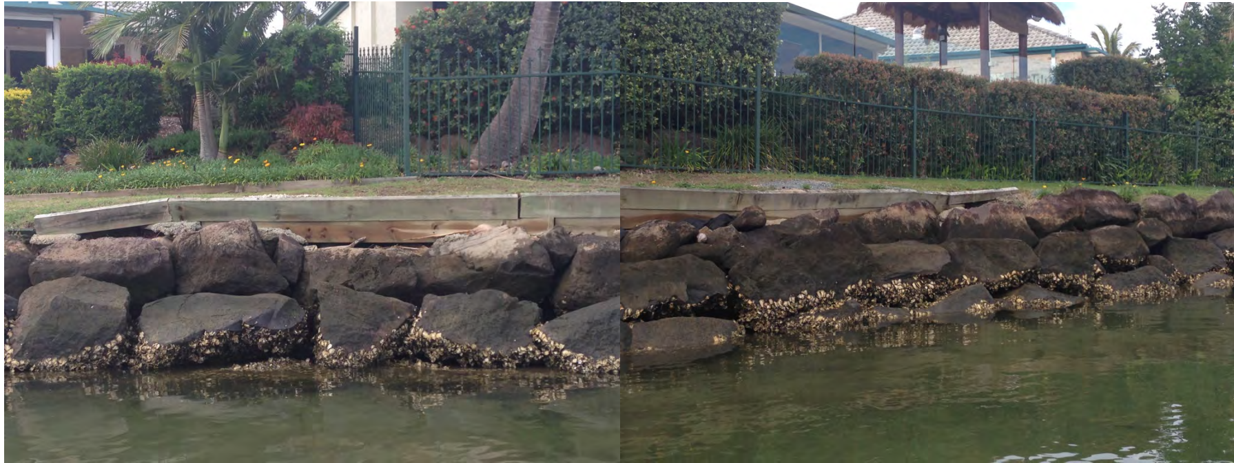
Plate 3: View looking east showing the approximate extent of proposed rock revetment repairs (to be performed using barge mounted excavator in adjacent Terranora Inlet)
