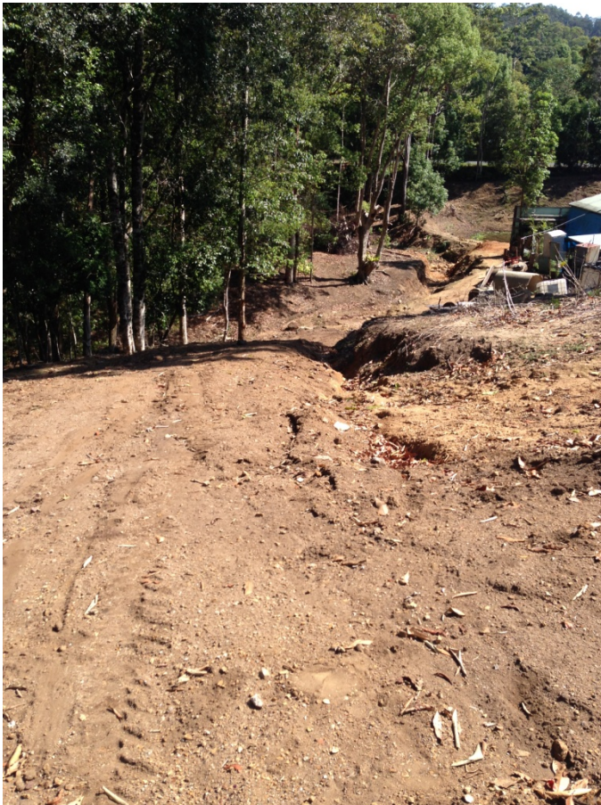
Photo 2 - Drainage line adjacent to water course that improved sediment and erosion control practices were identified to be established.
